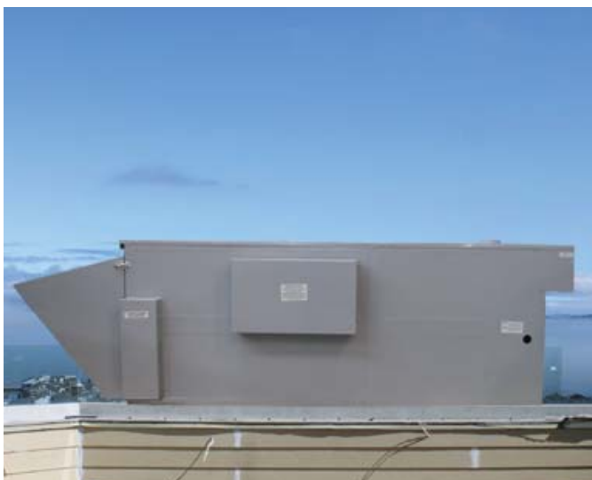
Readily accessible control panel and actuator
